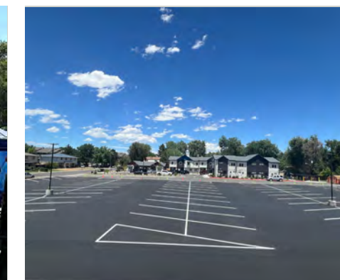
Work was delayed due to rain on June 25, but work continued once the weather passed. We now have a newly paved and striped parking lot!
