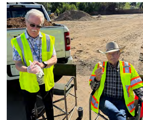
Rod Edmonds (left) and Butch Howard (right) directing traffic on a Sunday while the parking lot work was ongoing.
