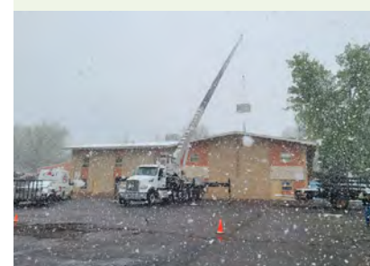
The new Education Wing A/C units being installed during the snow storm.
